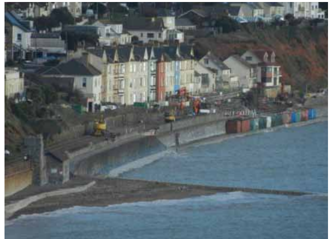
View of the repairs at Dawlish in winter 2014 - notice the sea containers lined up to protect the wall Pat Wilson © RGS-IBG Discovering Britain
