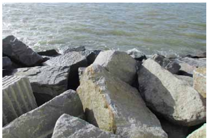
Some of the rock armour used to strengthen the sea wall Rory Walsh © RGS-IBG Discovering Britain
