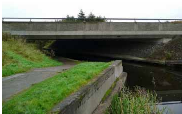
M80 bridge over the Forth and Clyde Canal near Banknock © Gordon Brown, Geograph (CCL)
